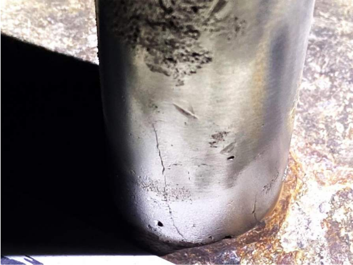
Severity level 3, visible cracking, and severe pitting
