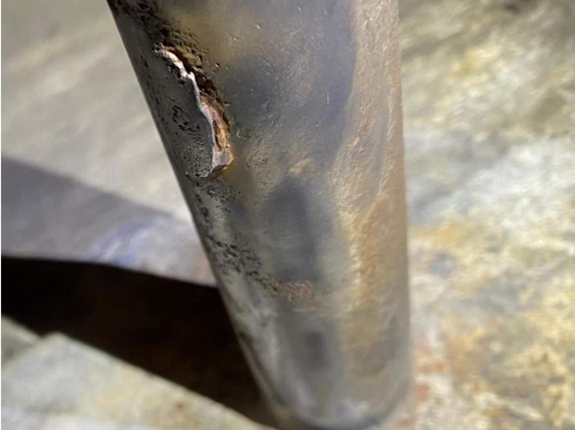
Severity level 3, visible cracking, and severe pitting
