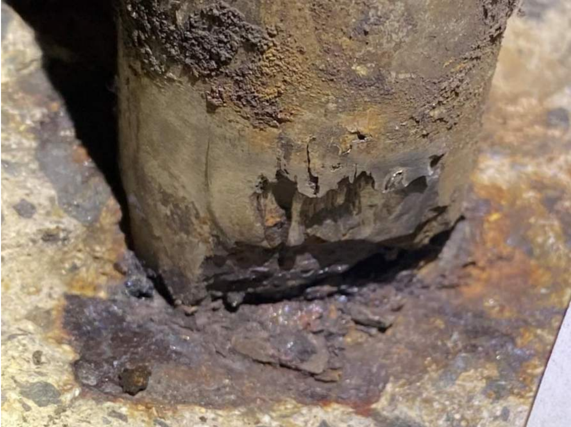
Severity level 3, interface fracture and severe corrosion
