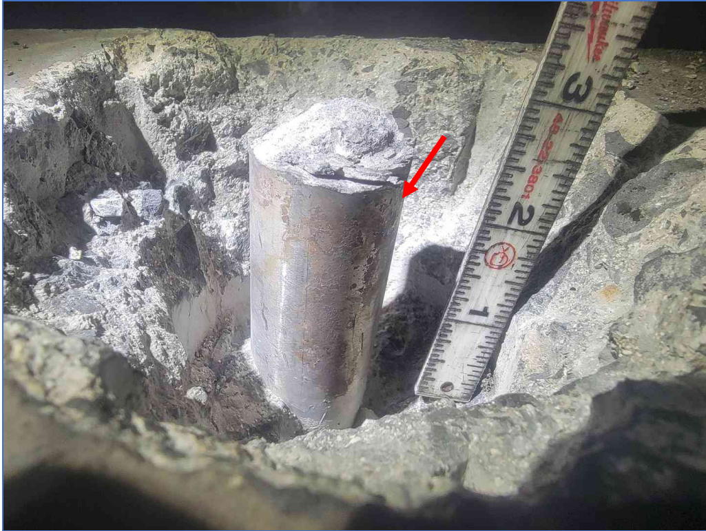
Photo 5: Fractured rod with corrosion in the top 2 in. (Rod 41, inbound bore, Kaneohe side).
