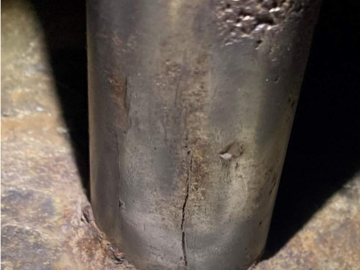
Severity level 3, visible cracking, and severe pitting
