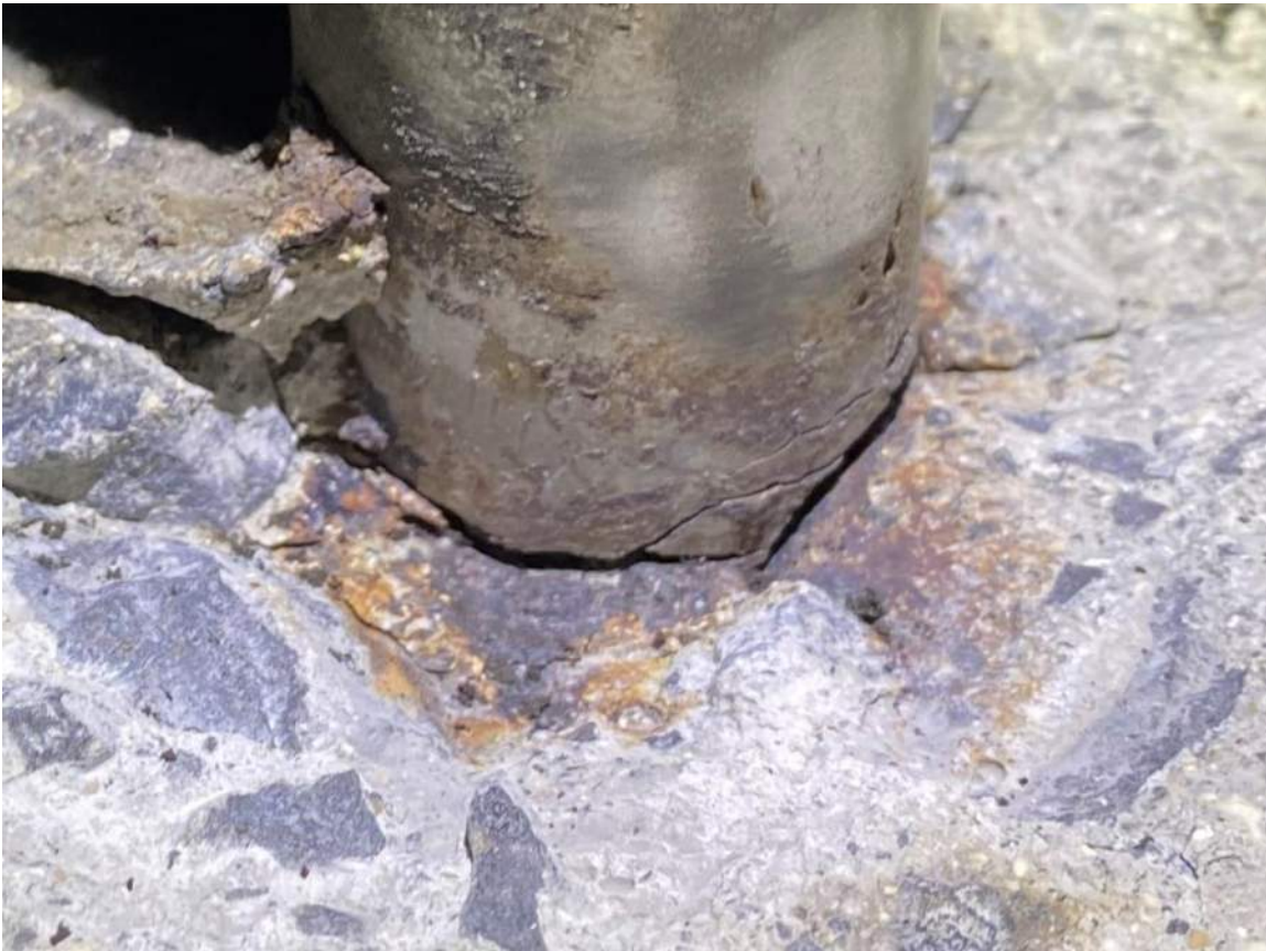
Severity level 3, interface fracture
