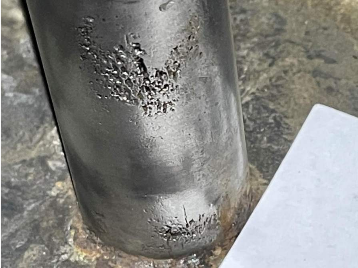
Severity level 3, visible cracking, and severe pitting
