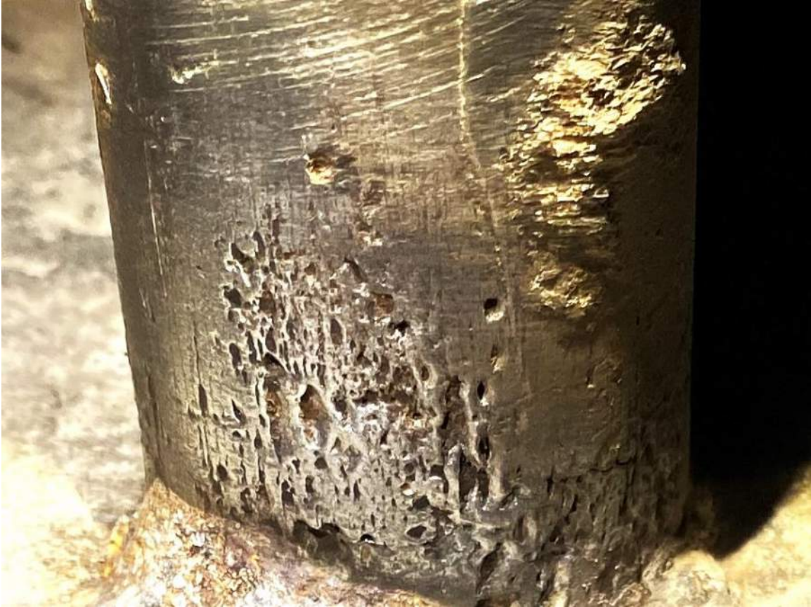
Severity level 3, visible cracking, and severe pitting
