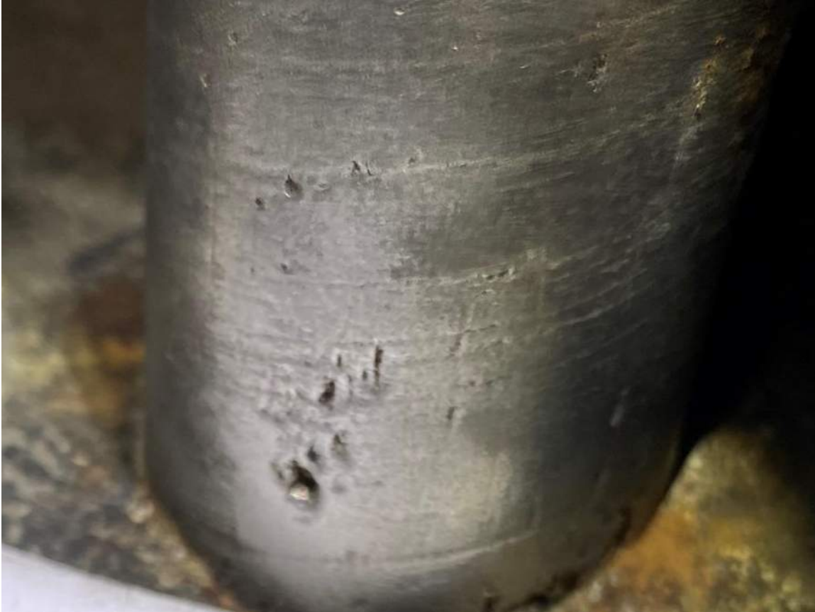
Severity level 2, moderate pitting
